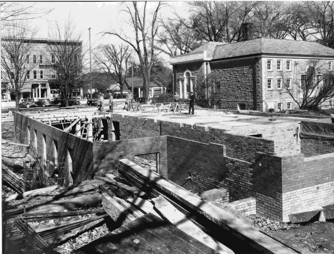
Construction of the new post office in Granville (left, and below) began during the fall of 1936 and was completed during the early summer of 1937.
